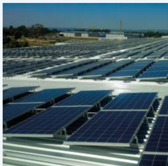
Solar installations on all new group builds.
